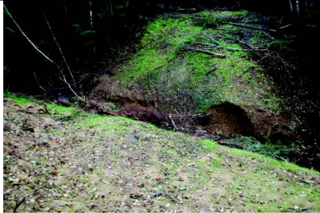
Photo 7. Representative culvert removal and road decommission site at tributary to Pole Creek, in Upper Pole Creek Basin.
