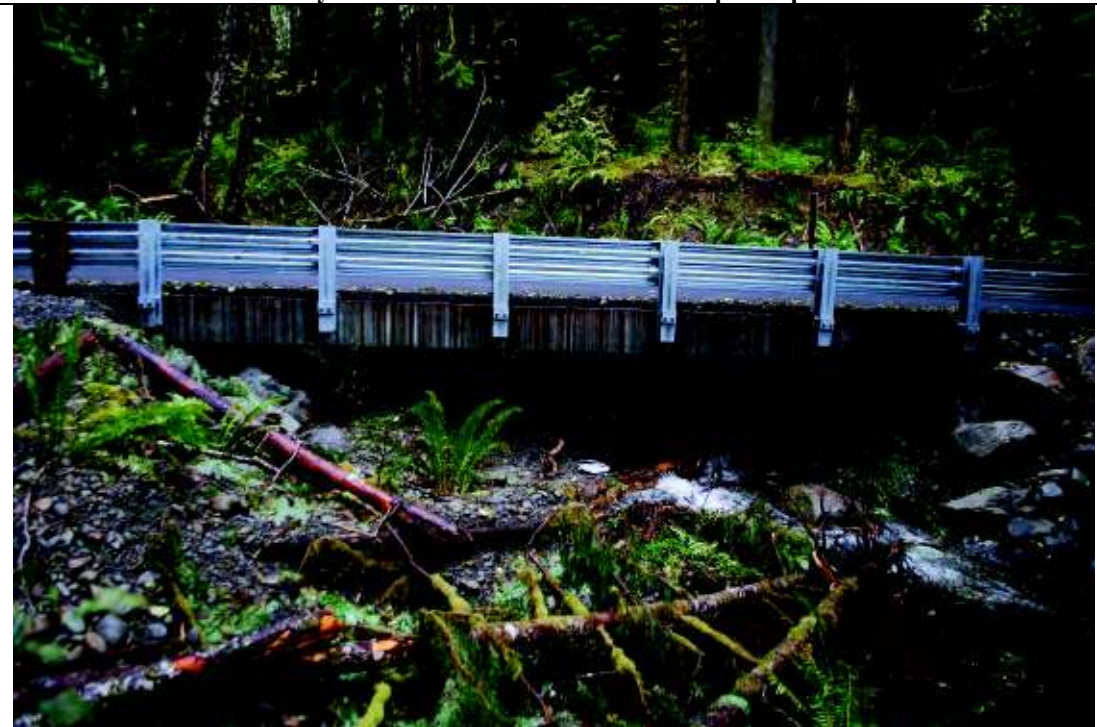
Photo 2. New Upper Hoh Road cement bridge over Pole Creek, in HRT's Spruce Creek Unit.
