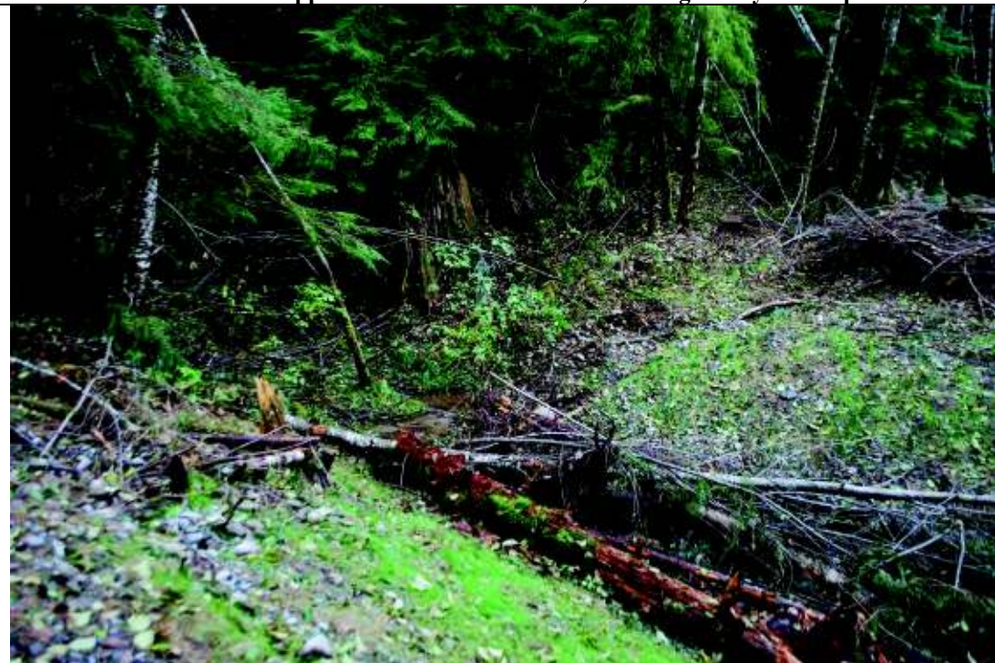
Photo 6. Representative culvert removal and road decommission site at tributary to Pole Creek, in Upper Pole Creek Basin.
